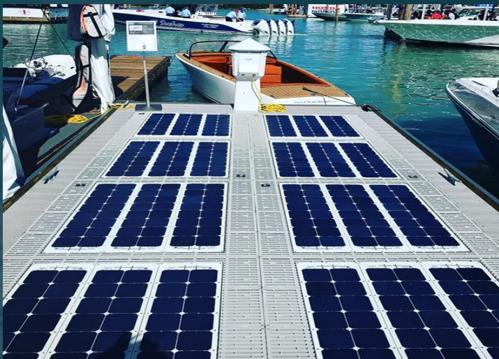
Solar Microgrid Docks
